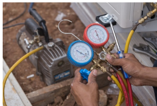
Fig. 5.5.12: Measuring pressure using manifold gate
