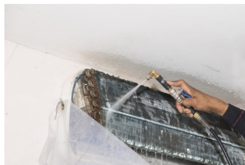
Fig. 5.5.9: Cleaning the indoor unit
