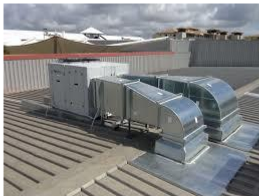
Fig. 7.1.3: Ductwork in package AC unit
